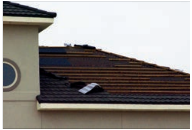
Figure 7. This residence had metal shingles that simulated the appearance of tile. The shingles typically blew off the battens, but some of the battens were also blown away.
